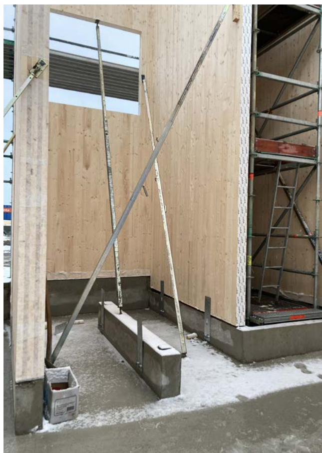
Wall elements raised on a concrete plinth with a damp course between them.
