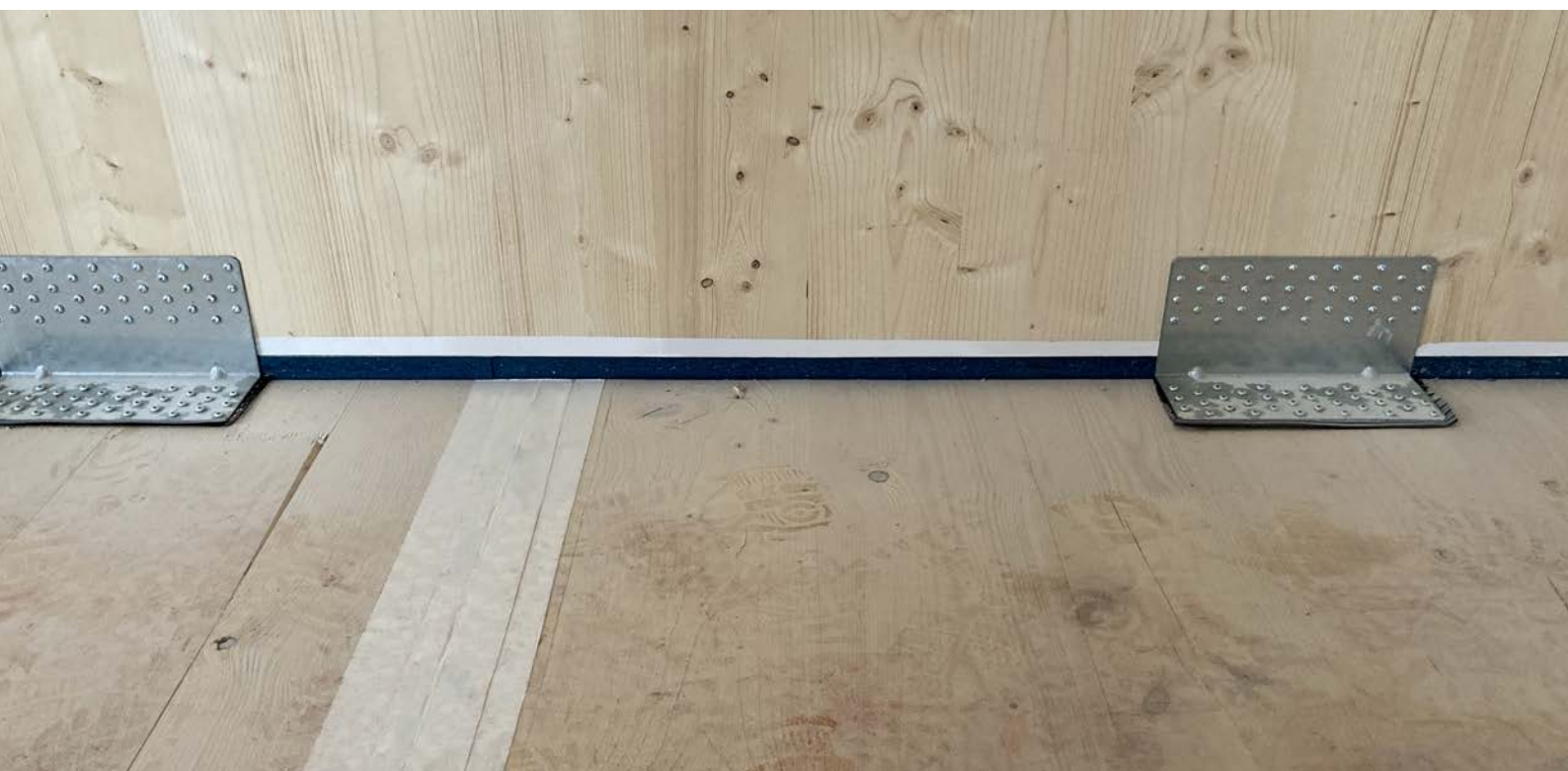
Taped joint between floor elements and where the floor meets the wall.
